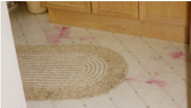
Photograph 4: Vinyl Flooring —Pink spots due to moisture problems arising from the impermeability of the vinyl flooring and ventilated and insulated crawlspace underneath.
